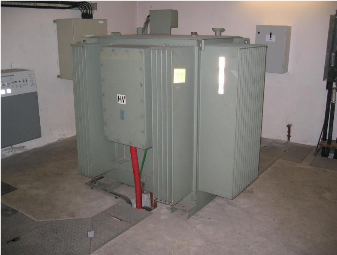
Photo 1 Transformer inside Transformer Room
