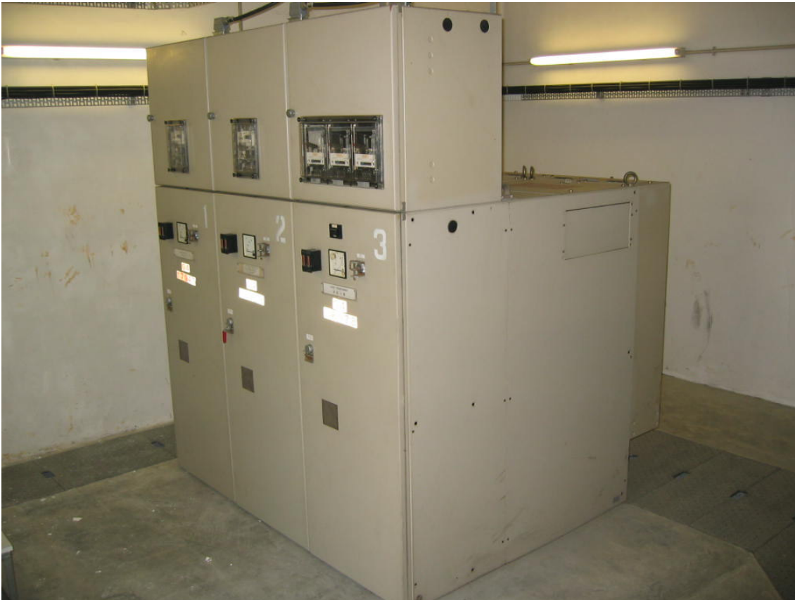
Photo 2 Electrical Panel inside Transformer Room
